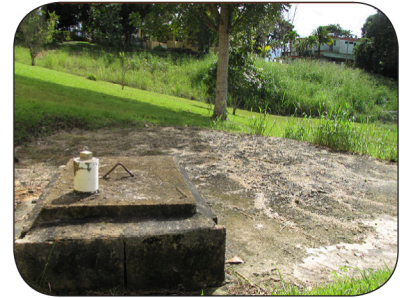
Keep septic tanks sealed.
