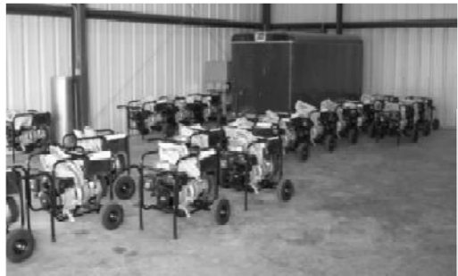
Small Generators and Fuel Camels
