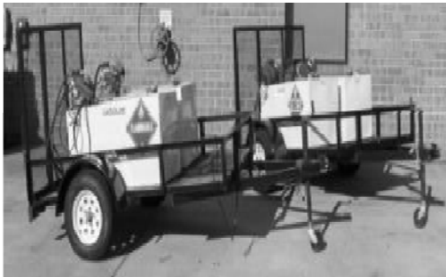
Small Generators and Fuel Camels
