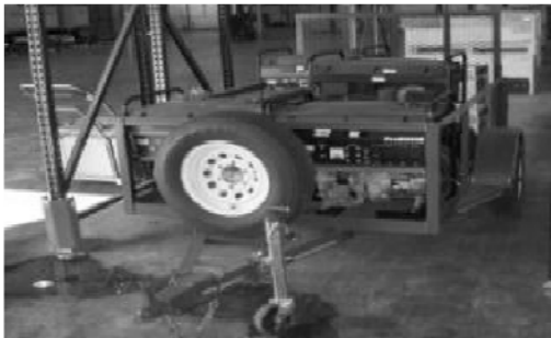
Small Generators and Fuel Camels
